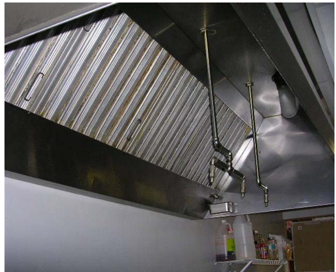
Fire ansul system
